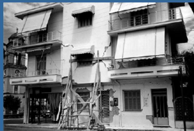
Fig. 25 Heavy infill damage, minor damage in R/C elements (YELLOW)
